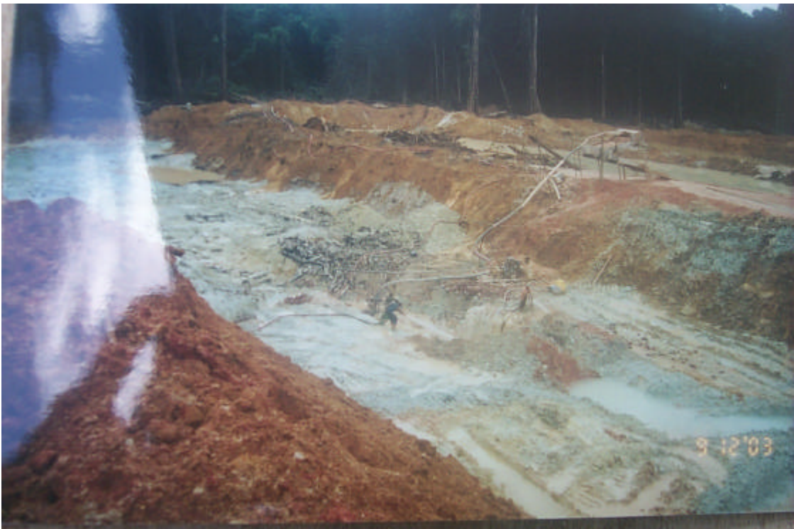
Photo 6 – Carlito's mining operations at Baramalli consisting of clean min pit, good pit definition and mine configuration and a closed-circuit recycle water system all totally enclosed within an outer perimeter dam.
