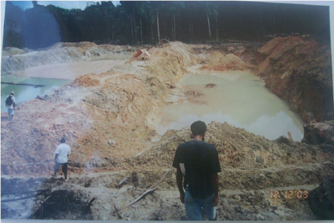
Photo 11 – Good pit configuration with, well defined pit faces at Araujo’s operation, Middle Aremu. Note, vertical pit faces (25 to 30ft.) deep with overburden Overcastted close to the edge of the mining face.
