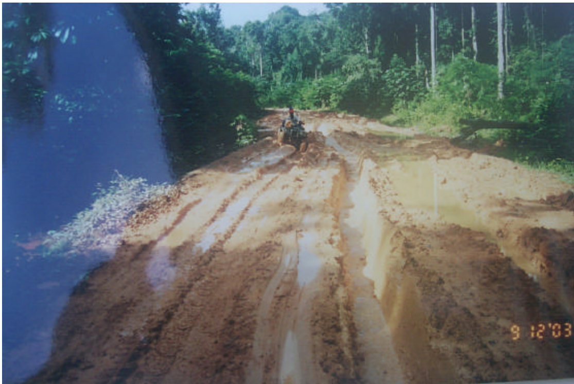
Photo 8 – The deplorable main access to route Baramalli.
