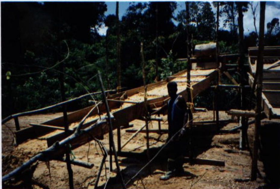
Photo 10 – Mr. Sherrif Standing Beside New Operating Sluicebox
